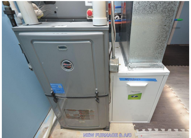
NEW FURNACE & A/C
